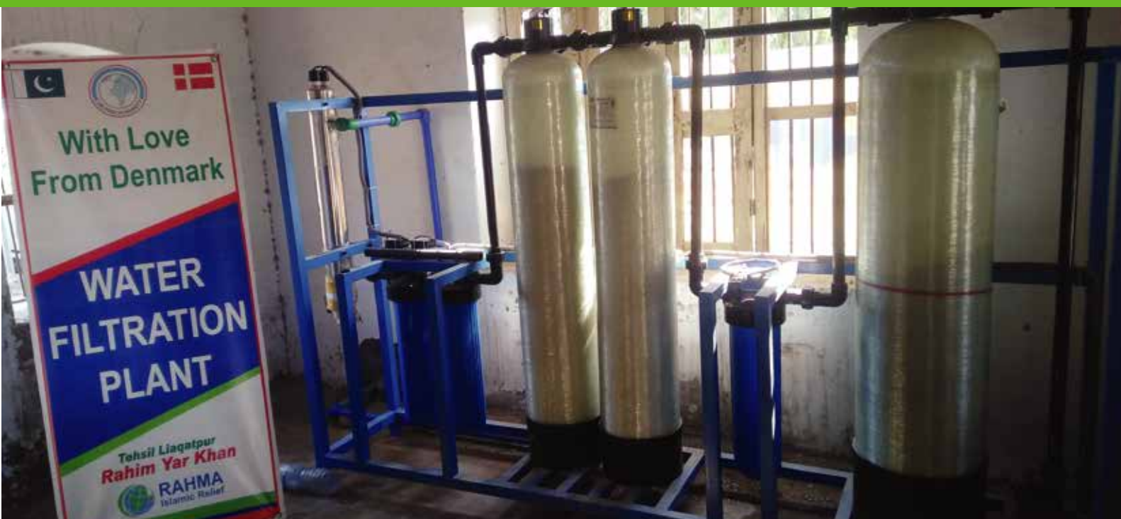
A newly installed Water Filtration Plant
